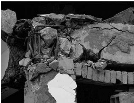
Gambar 1 Kegagalan Geser Sambungan Balok Kolom Beton Bertulang ( http://www.nbmcw.com/concrete/32646-seismic-retrofitting-of-rc-beam-column-connections.html )
