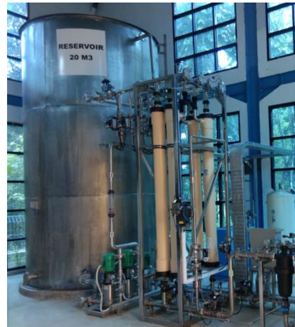
RESERVOIR KAP. 20 M3
