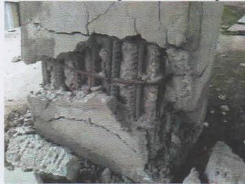
Fig. 2 : Main column failure, reinforcing bars undeformed.
