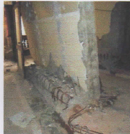
Fig. 3 : Thin column failure at the "core" area
