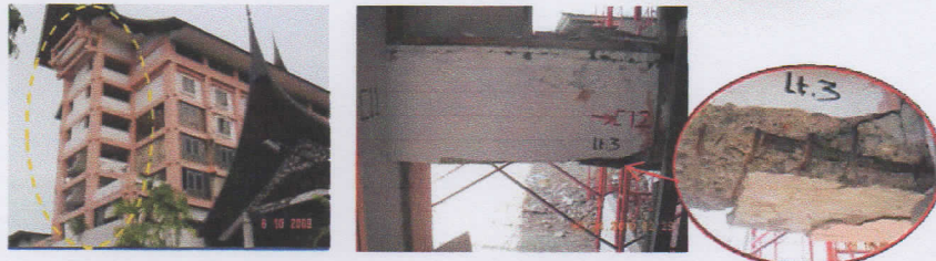
Fig. 6 : Beam damage at left-side stair shaft due to poor detailing and poor concreting
