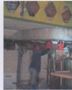
Fig. 15 : Jacking of concrete beams at the perimeter of core area to restore the original level
