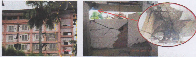
Fig. 5 : Beam damage at right-side stair shaft
