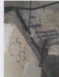
Fig. 4 : Beam failure, reinforcing bars not deformed
