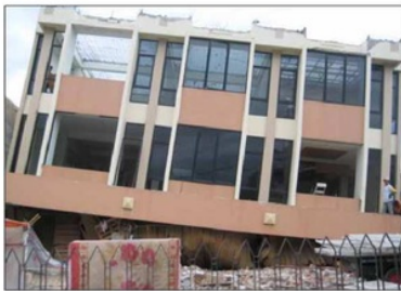
Fig. 1 Example of collapsed buildings; (a) A collapsed 3-story government building; (b) First story failure of a 3-story shop-house [1]
