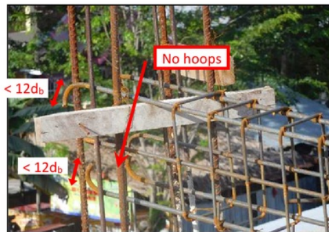
Fig. 24 Typical deficiencies in exterior beam-column joint
