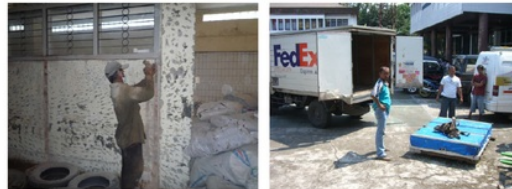
(a) Extracting Wall. (b) Transporting Wall. Photo 4. Preparation of Brick Wall Specimen
