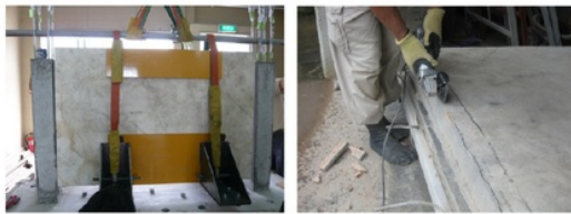
(a) Installing Wall. (b) Cutting off Wall. Photo 5. Installation of Brick Wall
