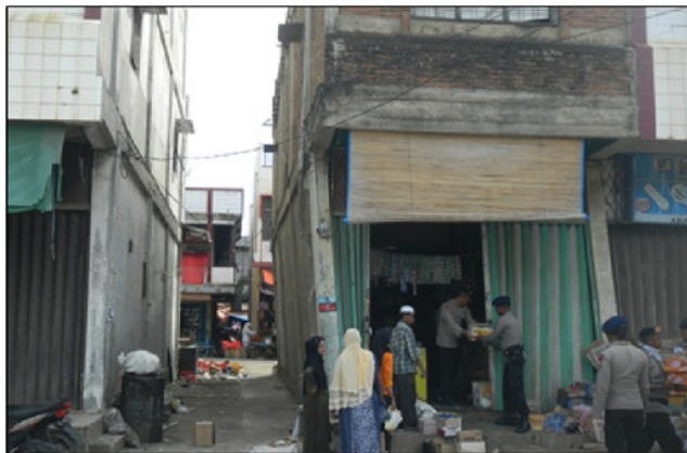
Figure 2 Soft-story effect on R/C frame structure
